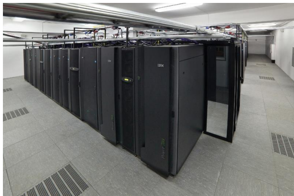
Figure 5. Inside a data hall.
